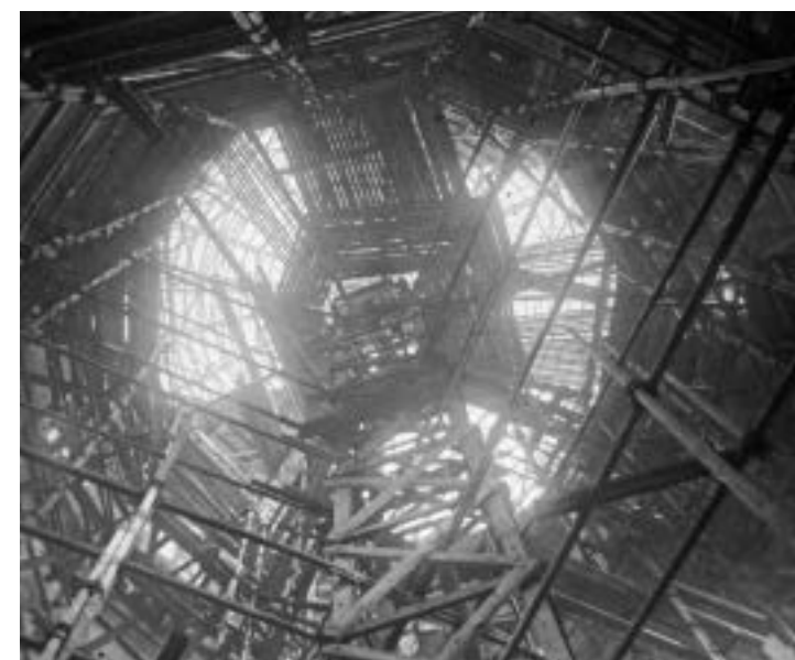
Four Courts, view of scaffold in main hall, 1926 IAA T.J. Byrne Collection, 2012/51.2/46
